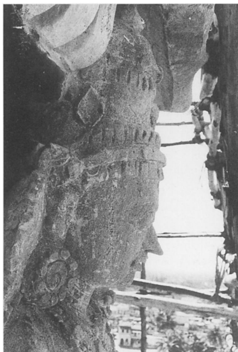
Fig. 5 - Noble and delicate moulded plaster detail (greater than life size) revealed by stripping away illicit surface overlay.
